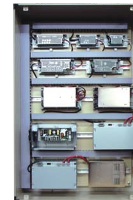
Mounting image inside Control panel
