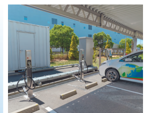
■Multi-EV charging system in Hanshin Factory
