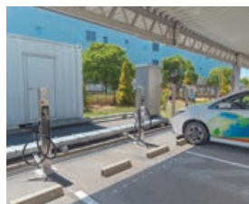
■ Multi-EV charging system in Hanshin Factory
